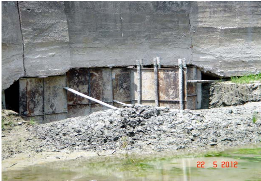
Photo-1: Deteriorated condition of damaged Borhar Khal in Polder 41/7B. Still sheets have been placed with support. No activity was noticed in the rehabilitation of the critical structure.
