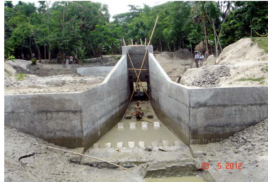
Photo-6: Construction of new Gholaghata regulator in Polder 39/1D. The progress is satisfactory.
