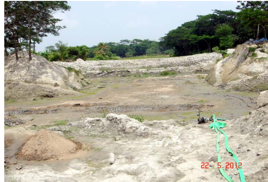
Photo-2: Almost abandoned condition of construction of additional new Borhar khal Regulator at Polder 41/7B.
