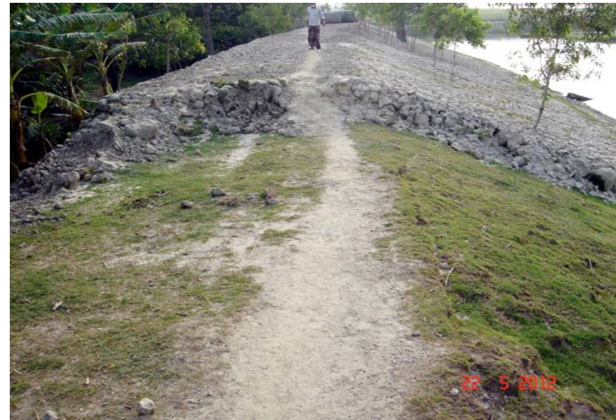
Photo-4: No base stripping has been done in the re-sectioning of embankment in Polder 42.
