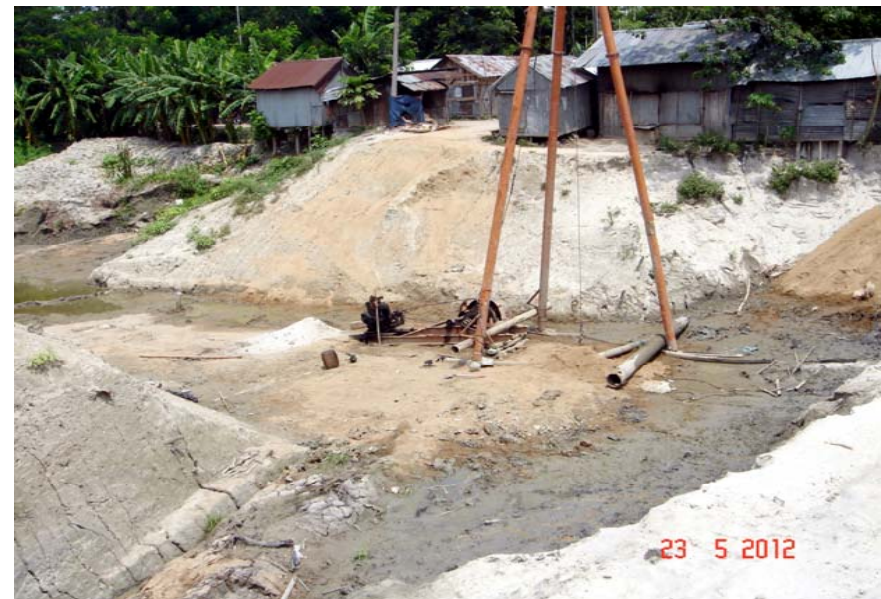
Photo-8: Poor progress of the new Bamna regulator adjacent to the Old Bamna regulator in Polder No.39/2A.
