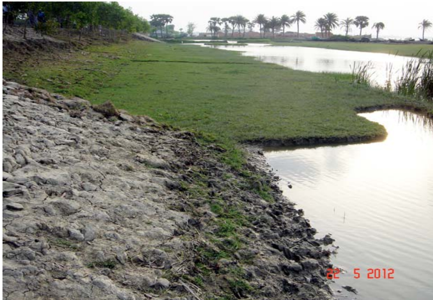
Photo-5: Designed berm width has not been maintained, instead existing berm has been spoiled in Polder 42.
