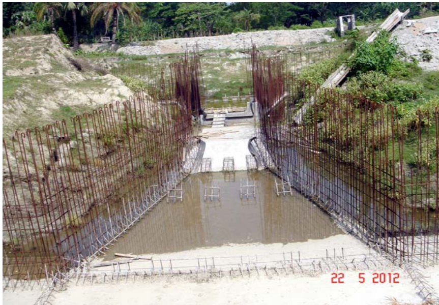
Photo-3: New construction of Napiter khal Regulator in Polder41/7B. The critical concrete work up to foundation level has been done. The site was found abandoned due to negligence of contractor.
