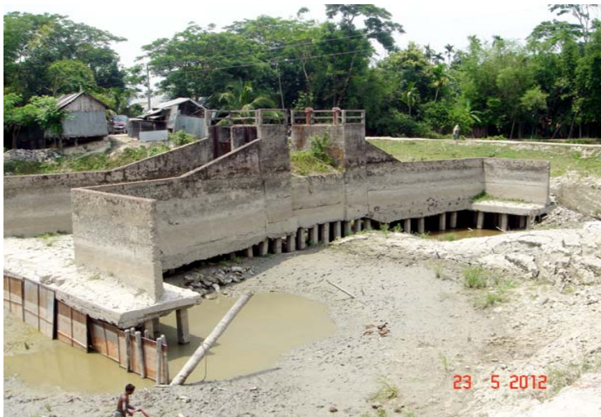
Photo-7: Deteriorated condition of damaged Old Bamna sluice in Polder No.39/2A. No activity in the field. Immediate rehabilitation is essential.
